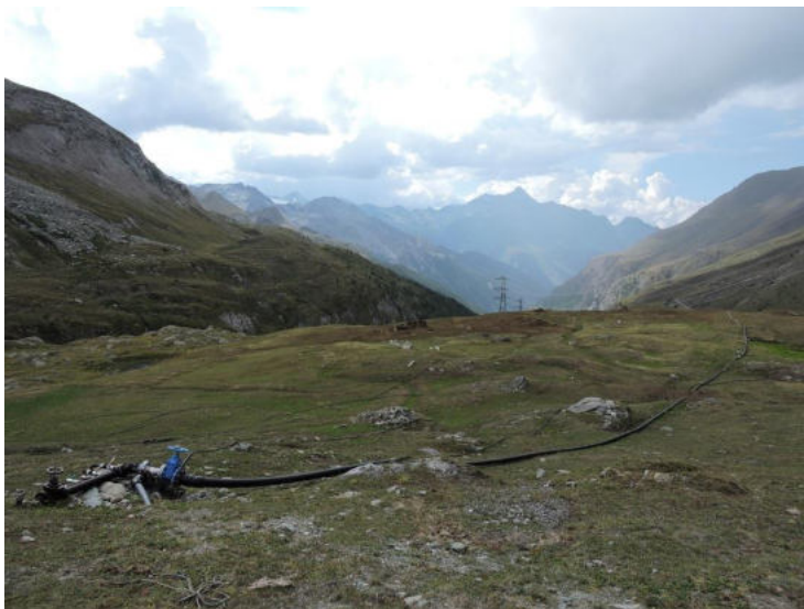
Pipes for fertigation, Aosta Valley.
