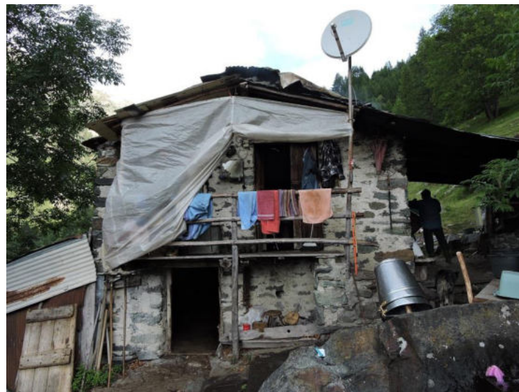
Need for structural interventions, Piedmont.
