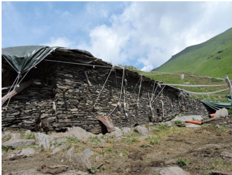
Alpage in use with serious structural problems, Piedmont.
